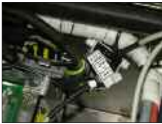
Figure 3: Example of current transformer for power measurement inside the HVAC system.
